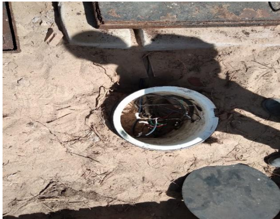
Sewer pump electrical junction
